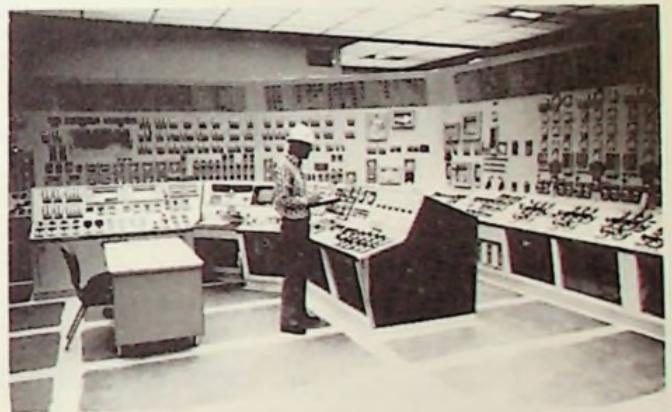
Control Room Diablo Canyon Nuclear Plant
